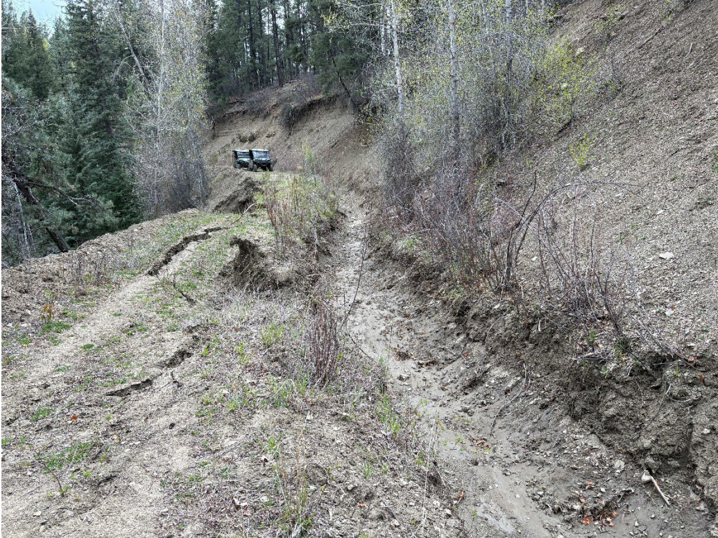
Ditch bank failure looking south, well maintained ditch on the right
