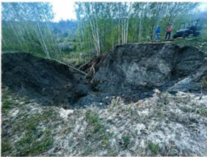
Photo of Breach #1: June 1, 2023
